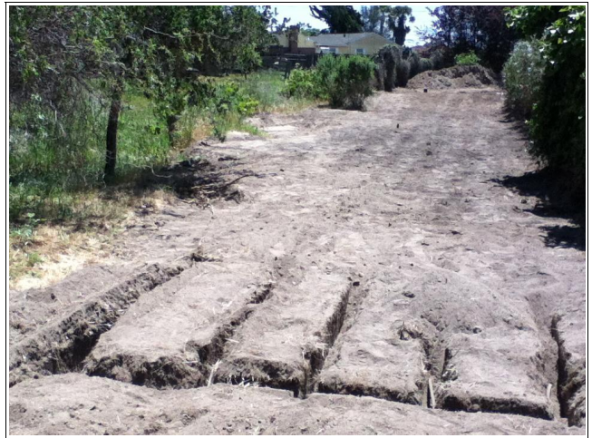
Geoflow subsurface drip system – approximately 500 sq ft
