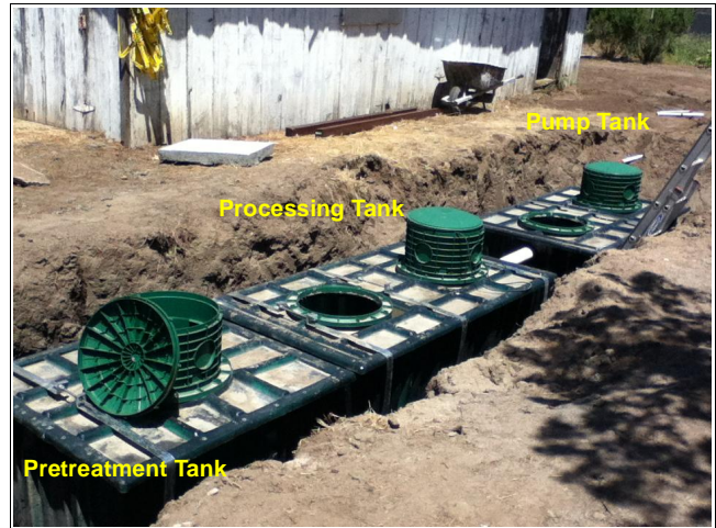
AK6S245F features a 424 gal pretreatment tank with 600 gpd processing unit; flows to separate 750 gal pump tank
