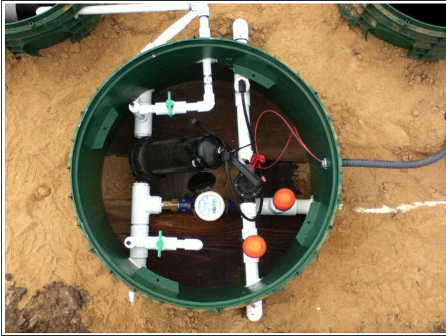
AquaKlear's headwork's manifold features a 120 micron disc filter, sampling port, flowmeter, solenoid valve & air-release valves (to prevent siphoning)
