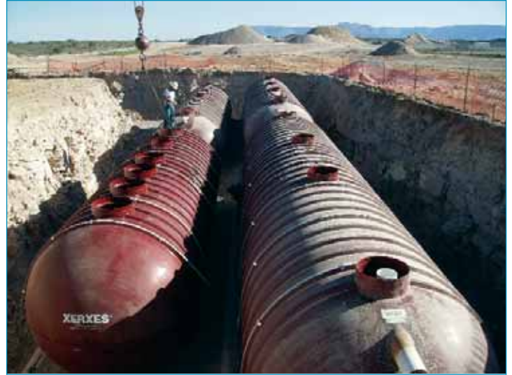
Tanks set in excavated bedrock
