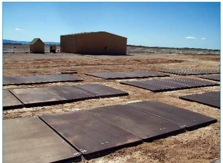
Advantex AX-100 treatment pods installed at grade elevation
