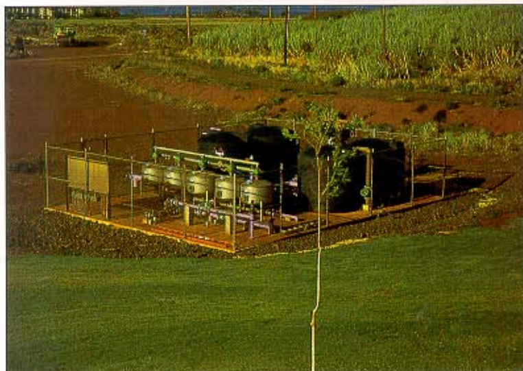
The central irrigation filter and distribution station at the Kukuila reclamation project provides water to turf and landscape plantings.
