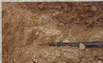
Figure 3: Root zone development around and along the dripline but not in proximity to the drippers
